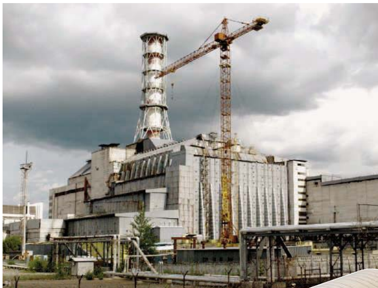
A sheltering sky. Work is about to start on a steel arch—the world’s biggest movable structure—to cover the disintegrating shelter now enclosing the ruins.
